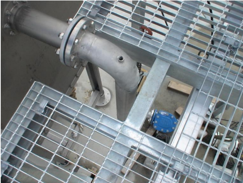
Figure 1.11 — Noise Source 11: Pipe/walkway contact. Fix: Isolate pipe from walkway.
