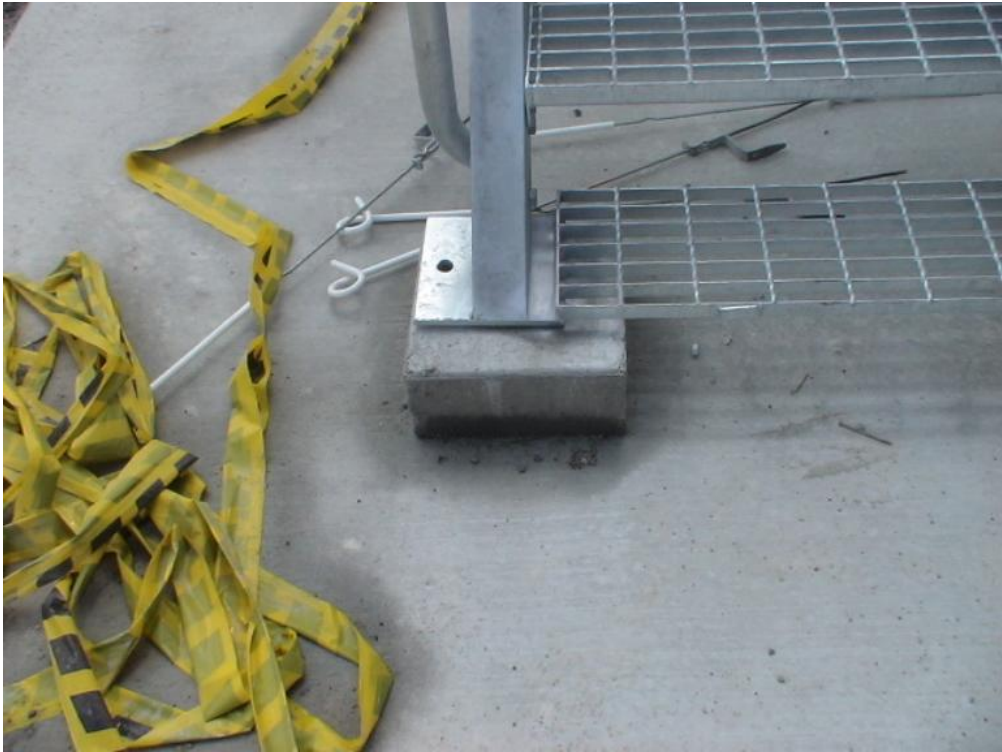
Figure 1.3 — Noise Source 03: Steel stair treads. Fix: Fill with polyurethane grout.
