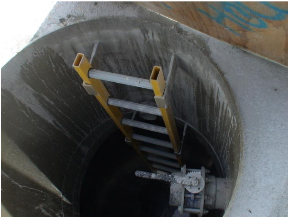
Figure 1.2 — Noise Source 02: Ladder resonance. Fix: Cap hollow ladder posts.
