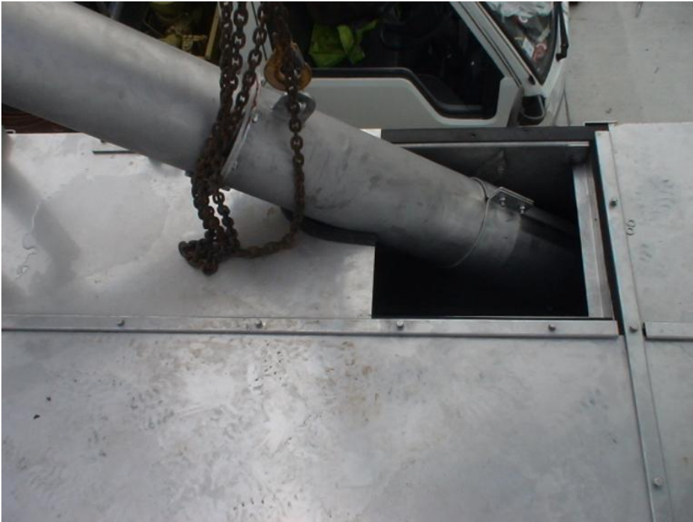
Figure 1.13 — Noise Source 13: Pipe isolation. Fix: Rubber isolation between pipe and unit.
