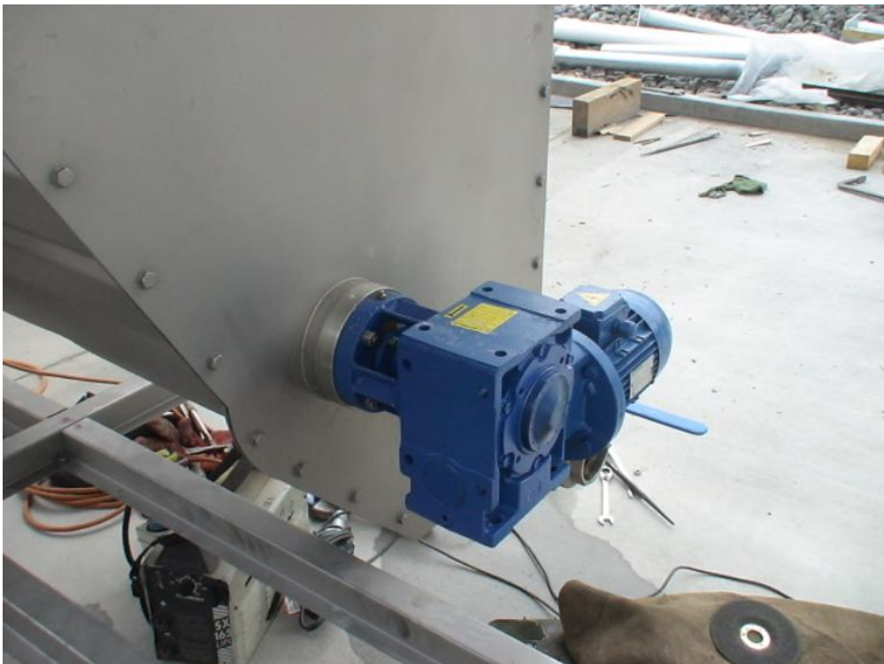
Figure 1.10 — Noise Source 10: Motor housing. Fix: Weld cancellation weight to high-node point.
