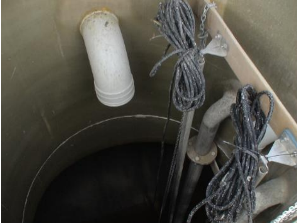
Figure 1.1 — Noise Source 01: Falling water. Fix: Lengthen pipe to reduce drop height.
