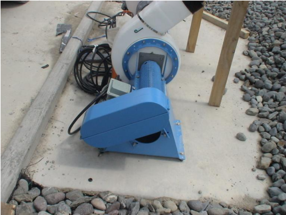
Figure 1.7 — Noise Source 07: Pump unit. Fix: Mount on springs; fill hollow base.
