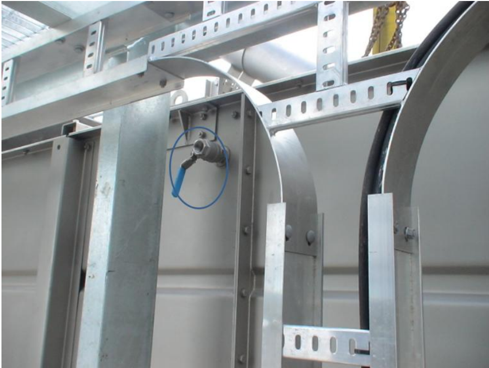
Figure 1.5 — Noise Source 05: Blower and casings. Fix: Flexible connector; fill casing holes.
