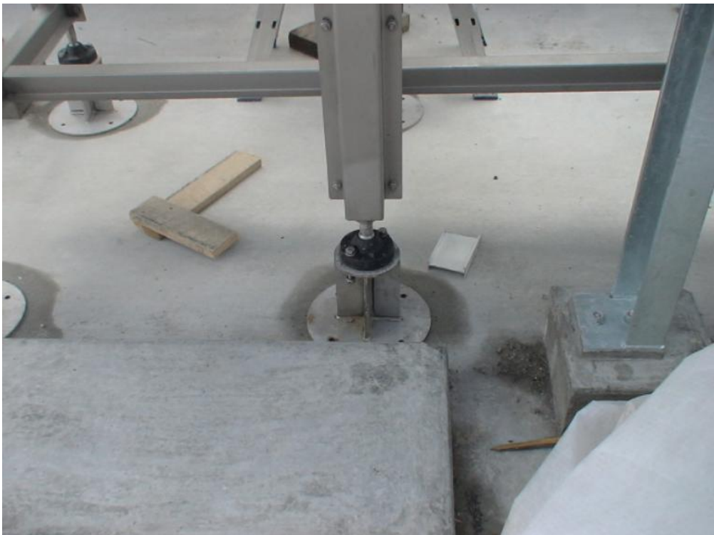
Figure 1.4 — Noise Source 04: Equipment feet. Fix: Ensure uniform load on all feet.
