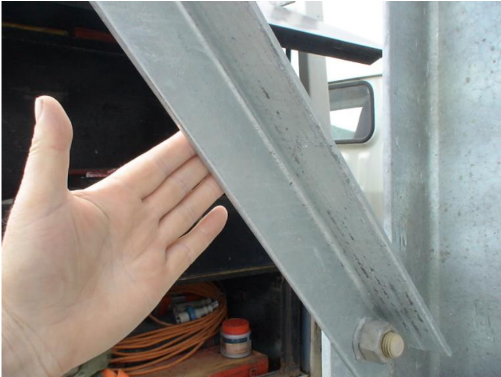
Figure 1.9 — Noise Source 09: Diagonal bracing. Fix: Isolate contact; add spring washer.
